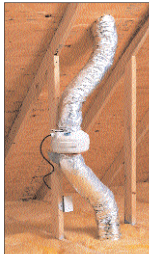
Typical attic installation
