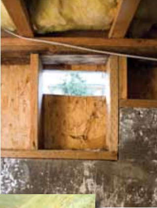
Mold growth on crawlspace foundation beams.
