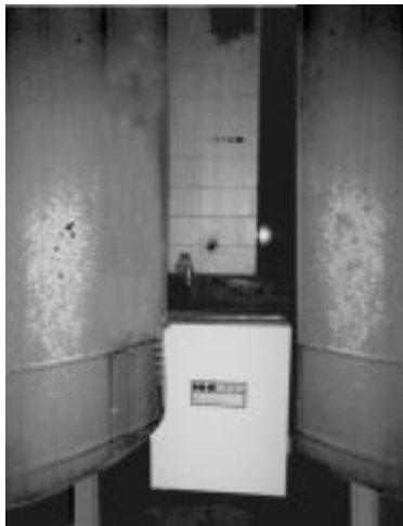
HI-E Dry 200 in water treatment facility
